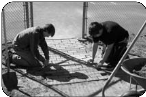
Patrick Edgerton and Chris Anderson work on a new entrance to the tennis courts.
